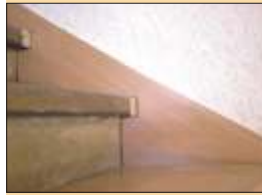
The string board will be cut out of a board, like a panel or polyester board, and just glued on.
